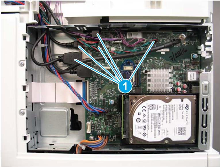
Figure 1-1201 Disconnect five connectors
