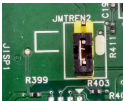
Interlock bypass enabled
